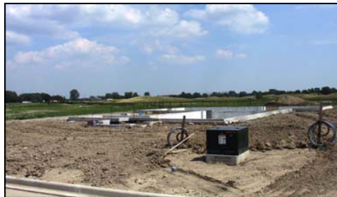
Construction of 3,500 sq. ft. ranch on lot 65 Only 22 single family lots still available.
